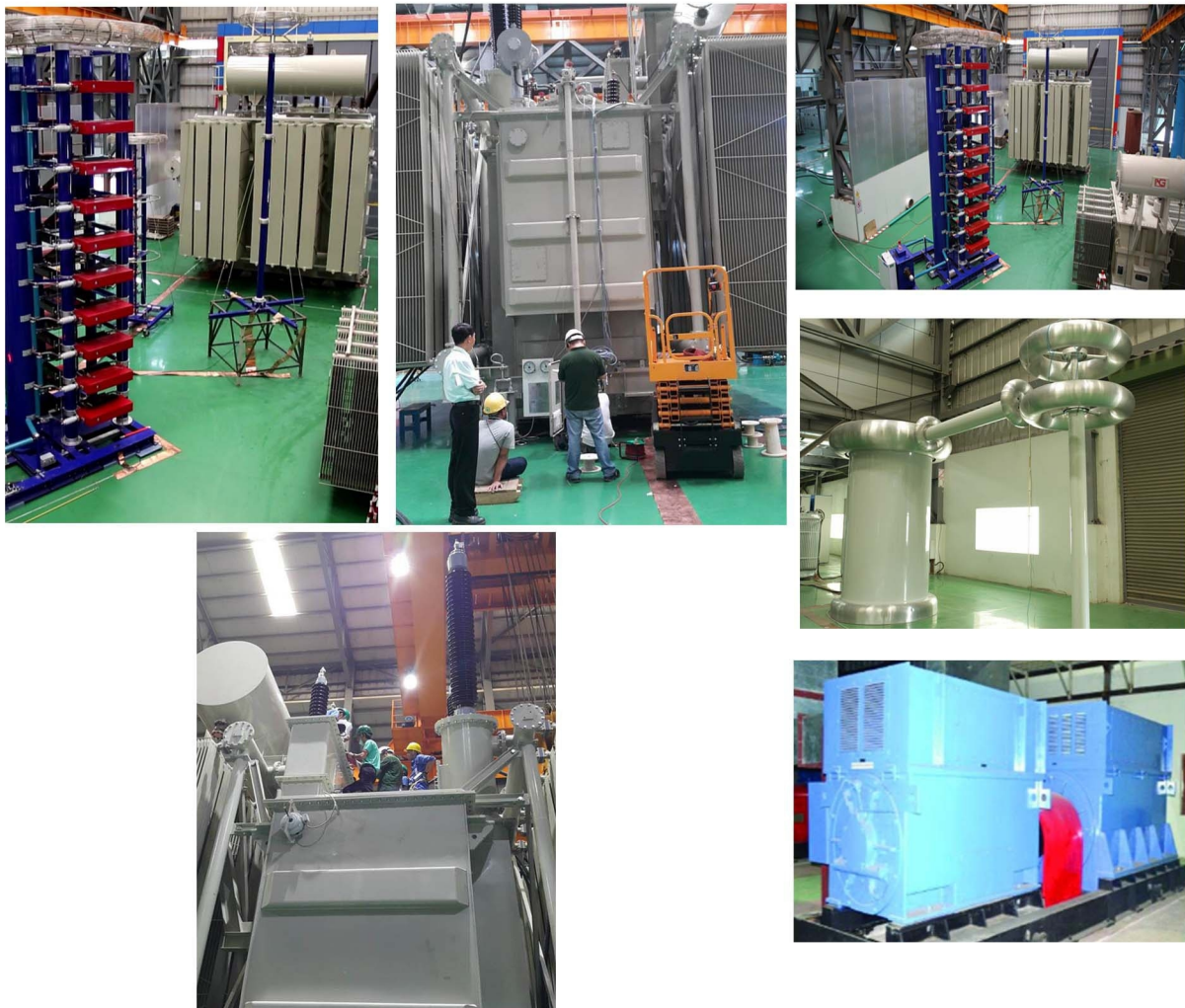
Extra-High Voltage Test Laboratory
